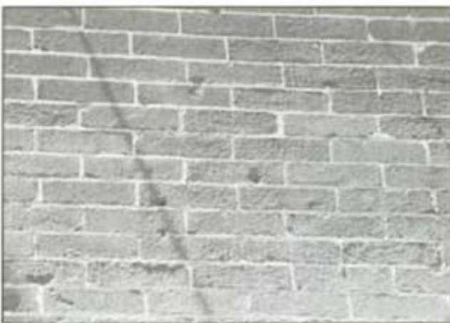
An eave overhangs this wall just a few courses above the top of the photo. The blasted bricks most exposed are "rotting" fastest.
