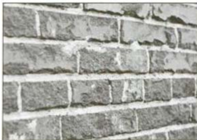
Sandblasting was the first crime perpetrated on these bricks. They were then repointed with a hard mortar -- speeding erosion.
