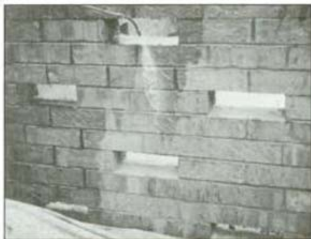
Applying a test patch of masonry sealer to brick in new construction. Photo courtesy of American Building Restoration.
